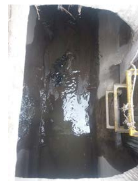
Figure 24 Typical stormwater drain where stormscous are deployed
